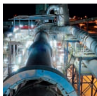
Clinker kiln at the Wazo Hill cement plant, Tanzania
